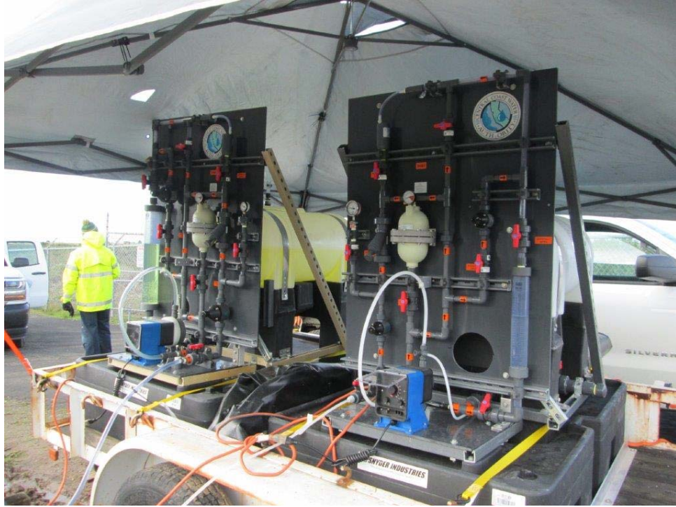
Tank 5 Inlet Vault Portable Chloramination Trailer, February 2022
