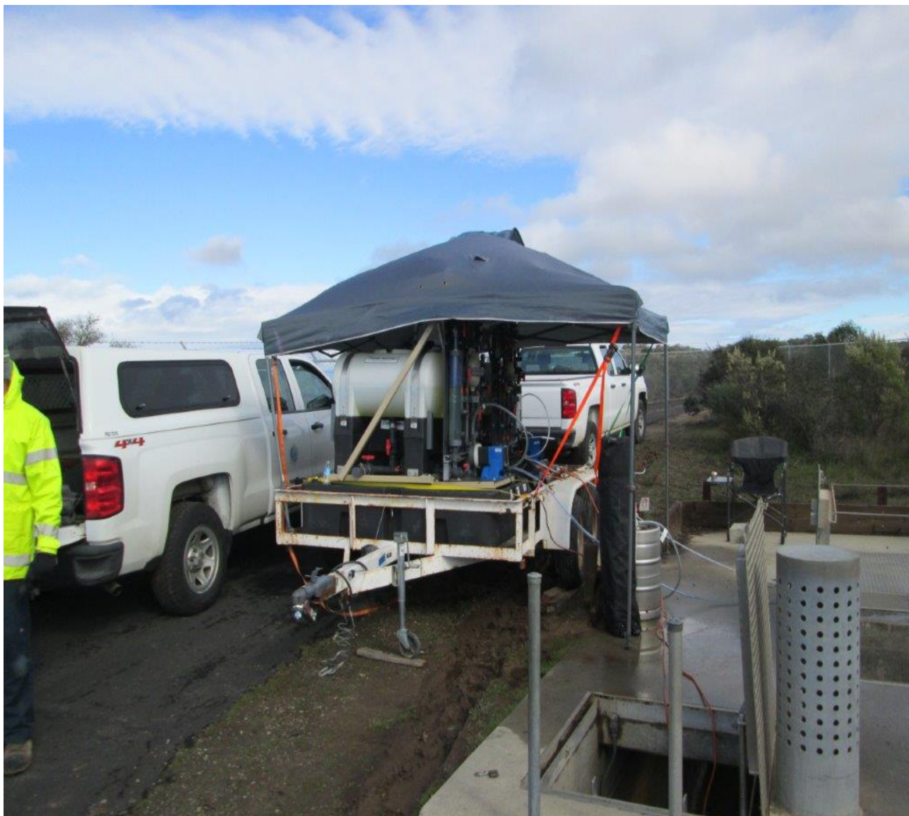
Tank 5 Inlet Vault Portable Chloramination Trailer, February 2022
