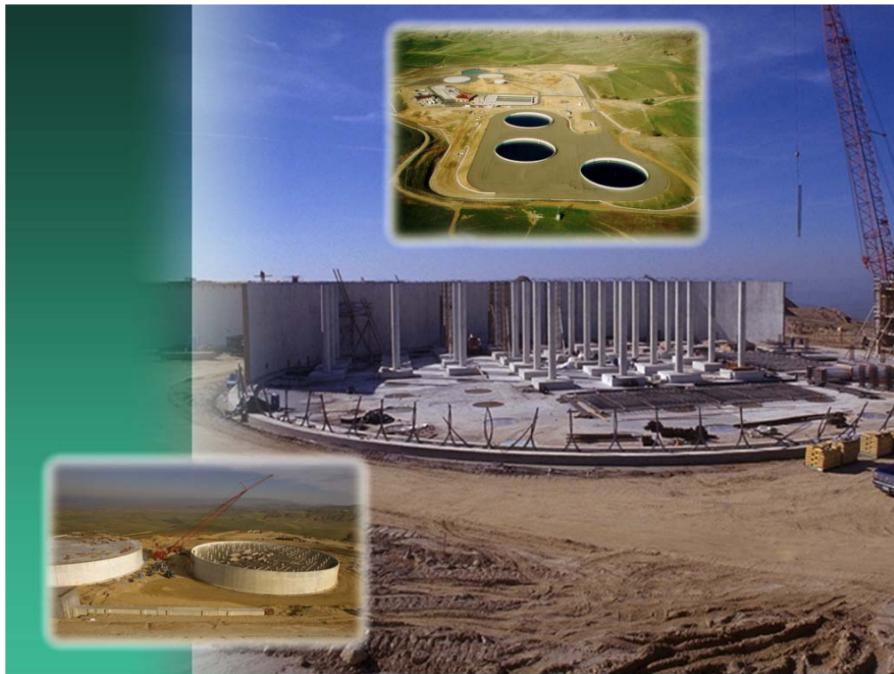
Top Insert: Tank 1 and Polonio Pass Water Treatment Plant site with raw water tanks in foreground. Above and left insert: Construction of treated water tanks with concrete roof-support columns visible inside the partially completed tank.
