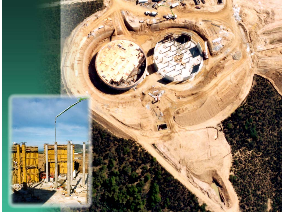
Above: Aerial view of Tank 5 during construction. Inset: Concrete pour of one of the wall panels with concrete column roof-supports in the foreground.
