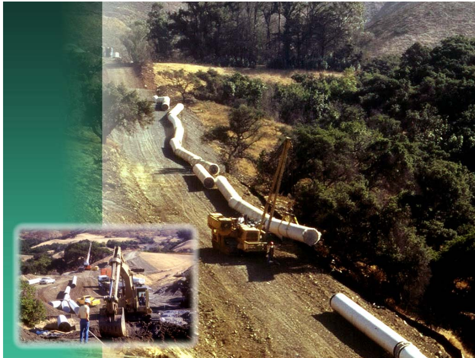
Above and inset: Construction by Valley Engineers of a section of Reach 5A1 that was redesigned subsequent to DWR's award of the Reach 5A1 construction contract to Homer J. Olsen. The redesign was required to mitigate impacts to oak trees and woodlands.
