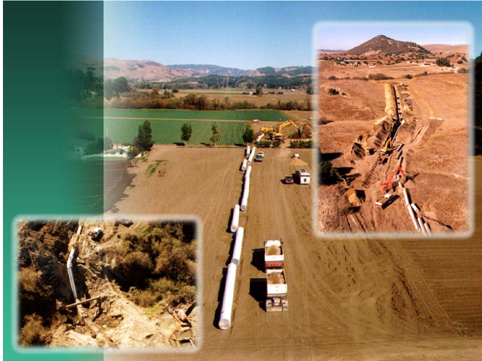
Right Insert: Pipeline construction in the Nipomo area, Pipeline Reach 5B. Left Insert: Construction of Tar Springs Creek crossing; temporary creek diversion piping crosses above the concrete pipeline encasement across the creek bottom. Above: Pipeline construction in Arroyo Grande area.
