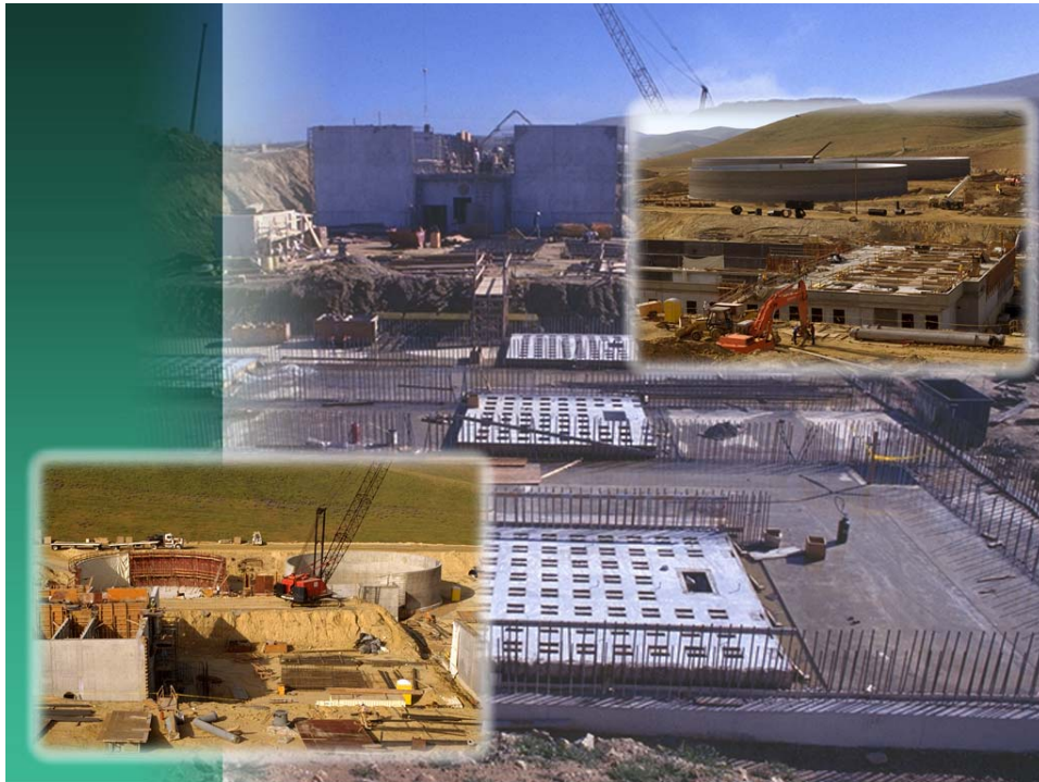
Right Insert: Foreground-construction of flocculation and sedimentation basins at the Polonio Pass Water Treatment Plant. Left Insert: Foreground-filter construction.
