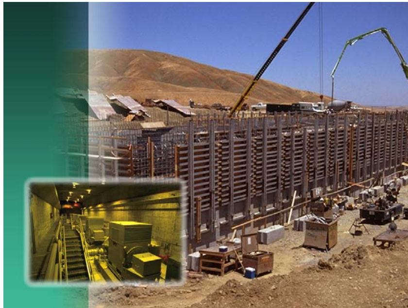
Above: Framing and pouring of concrete for the Blue Stone Pumping Plant wall. Inset: Interior of the Blue Stone Pumping Plant building housing six horizontal pumps and motors.
