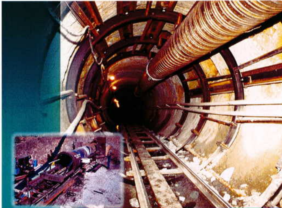
Above: Interior of 3,279' long Calf Canyon Tunnel prior to pipeline installation in Pipeline Reach 4. Inset: Calf Canyon Tunnel entrance.
