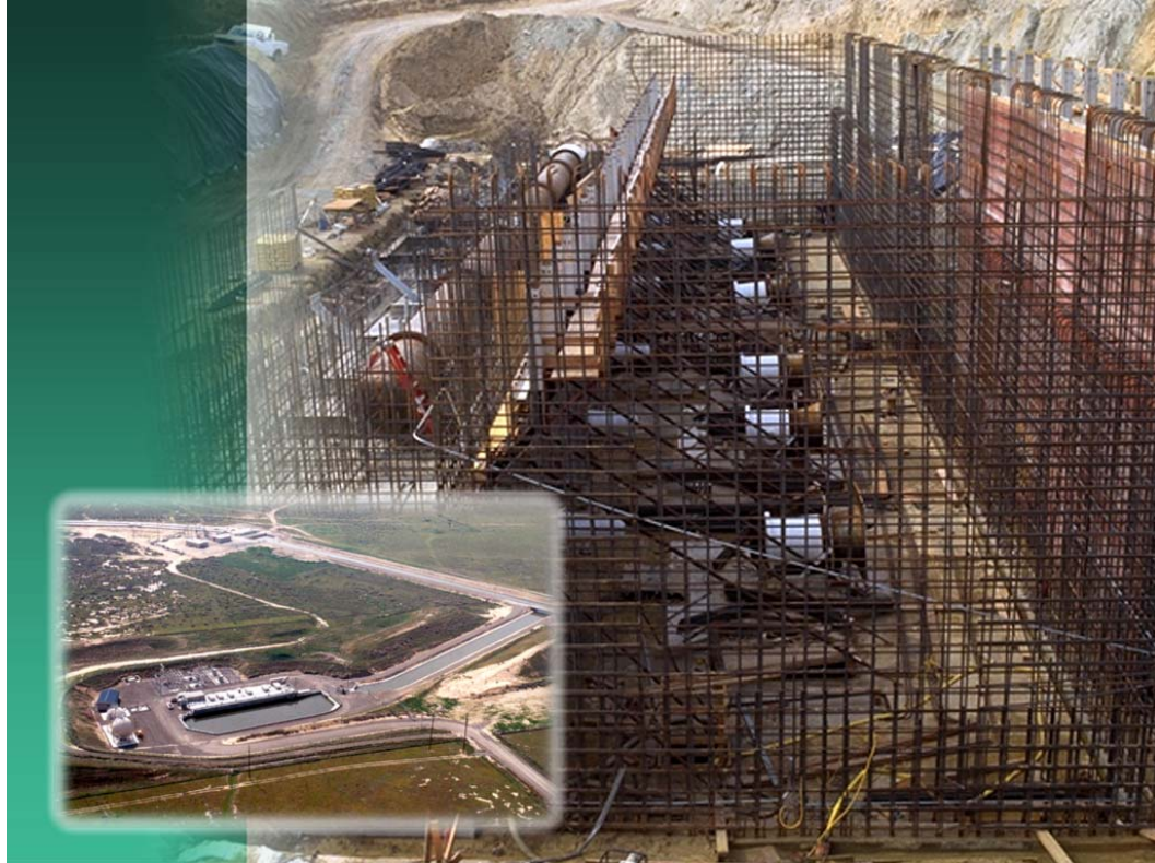
Above: Devil's Den Pumping Plant building wall reinforcement bars prior to concrete forming and pouring. Inset: Aerial view of completed pumping plant, inlet canal and Coastal Branch Phase I aqueduct in background.
