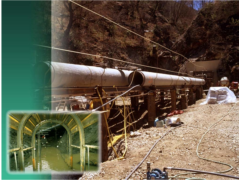
Above: Partially welded pipe sections prior to installation in the refurbished Cuesta Tunnel. Inset: Cuesta tunnel interior prior to refurbishment and installation of 42" diameter Coastal Branch Phase II pipeline and 24" diameter section of future San Luis Obispo County Nacimiento pipeline.
