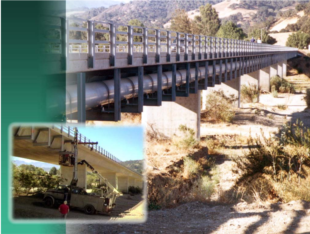
Above: Alisal Bridge crossing in Solvang. This is one of four locations where the pipeline is visible (i.e., not buried). Inset: Installation of pipe-support brackets on Alisal Bridge.
