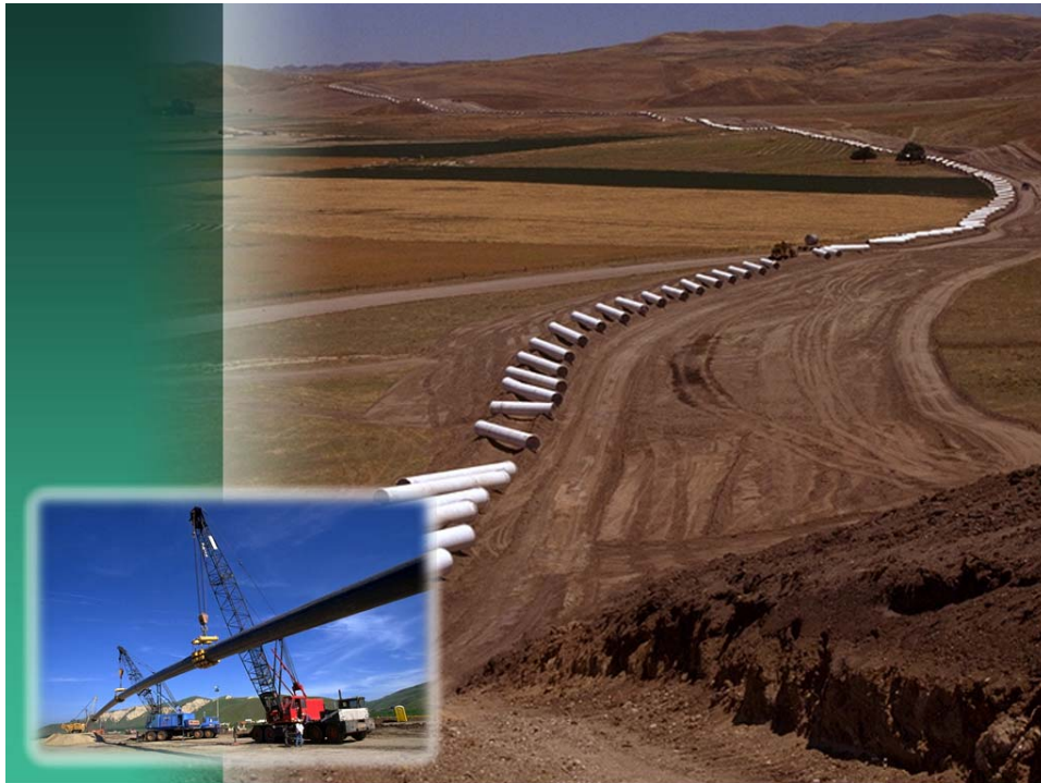
Above: Placement of 40' long pipe sections along the right-of-way prior to installation in Pipeline Reach 2. Inset: Installation of 1,975' long section of 42" diameter welded pipe through directionally drilled borehole under San Juan Creek.
