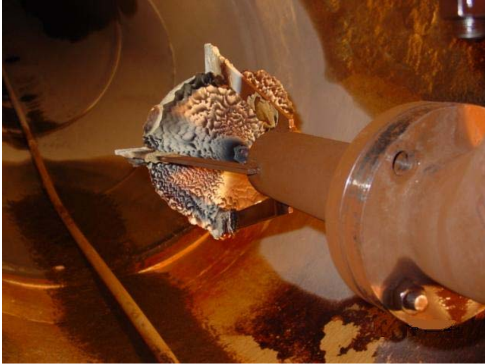
Chemical Injection Mixing Cone at Polonio Pass Water Treatment Plant.
