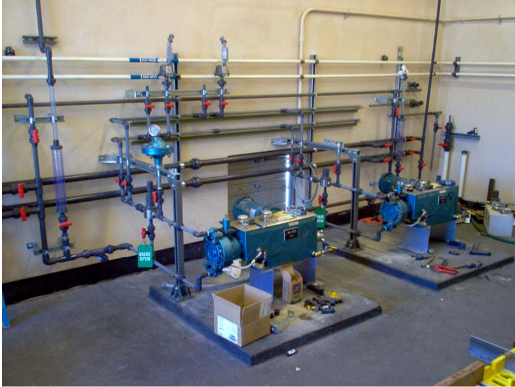
Rebuild underway on the Santa Ynez Pump Station Sodium Bisulfite Injection System.
