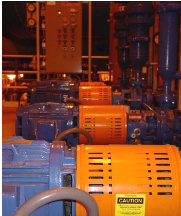
Utility water pumps at the treatment plant.
