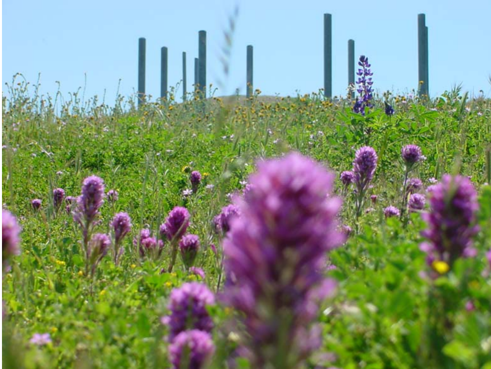
Air Vacuum Air Release Vault in Reach 1 below Polonio Pass Water Treatment Plant.
