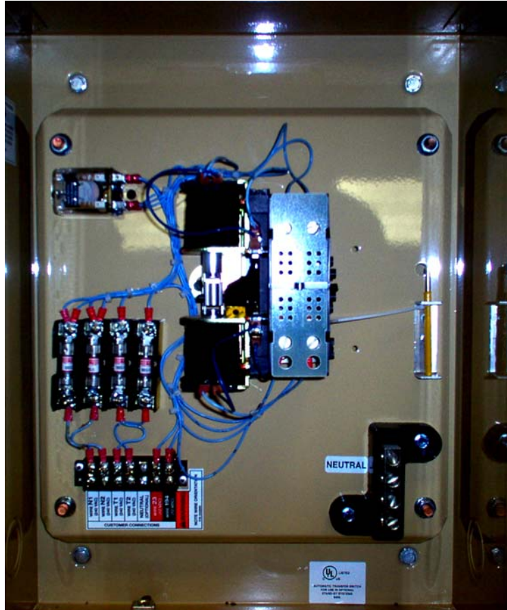
New Generator Transfer Switch at the Chorro Turnout.
