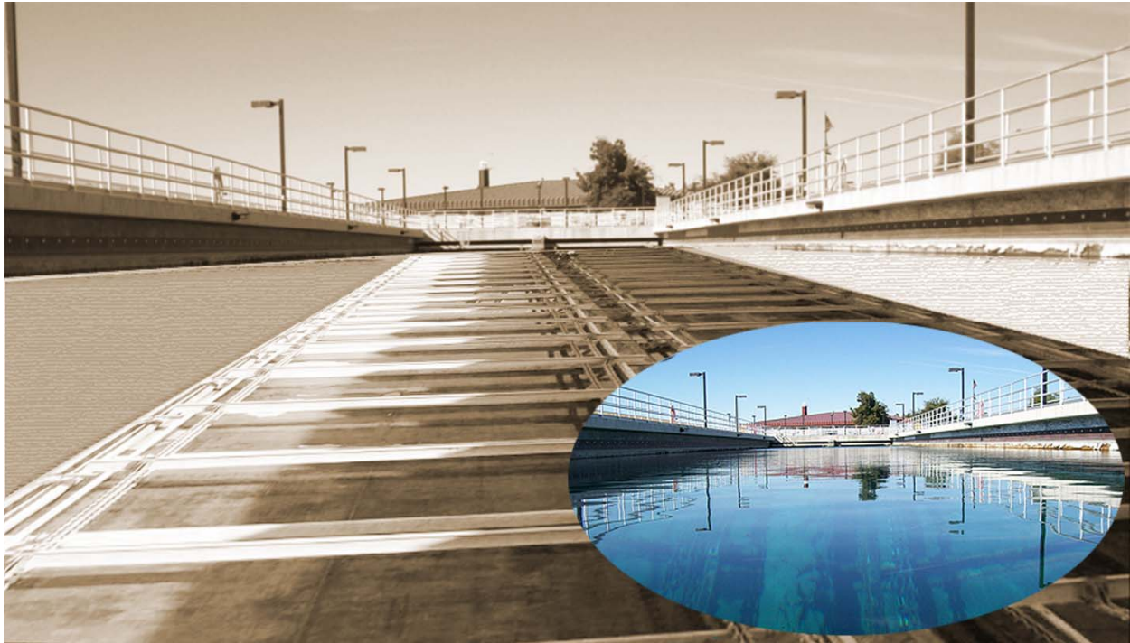
Sedimentation basin at Polonio Pass Water Treatment Plant
