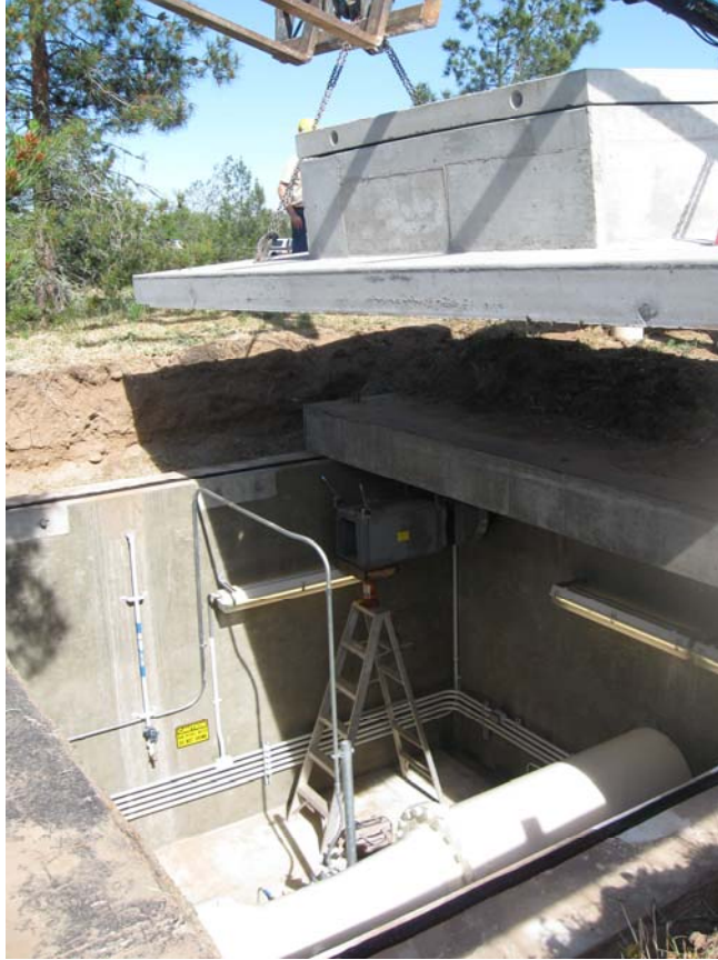
Santa Ynez Pumping Facility Station Outlet Vault
