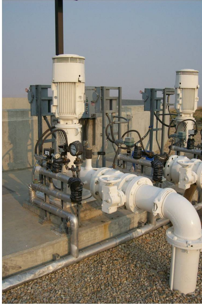
Waste washwater return pumps at Polonio Pass Water Treatment Plant
