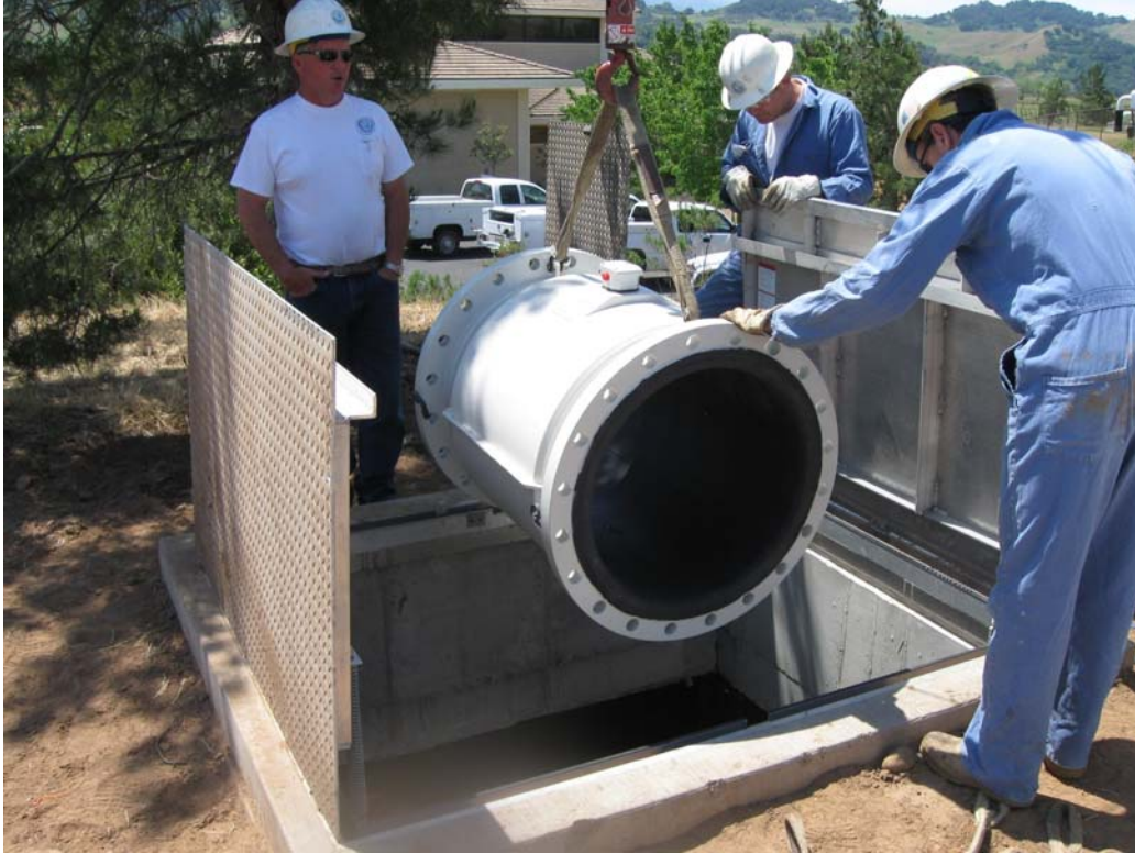
Installation of new outlet flow meter at the Santa Ynez Pumping Facility
