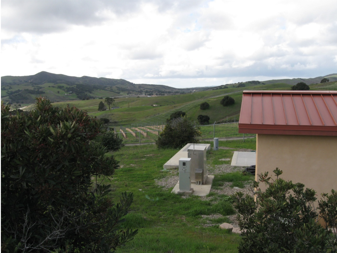
Tank 7 Remote Programmable Logic Panel
