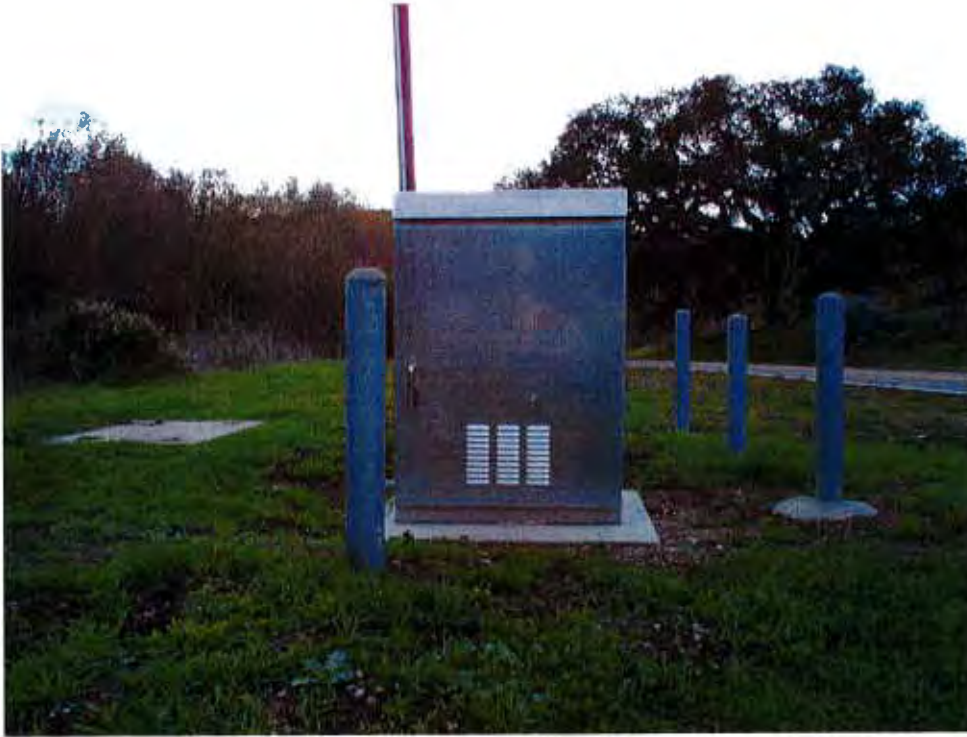
Isolation valve fiber optic pipeline control panel at Vandenberg AFB.
