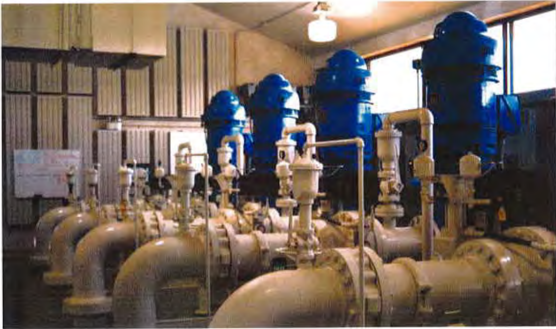
300 hp pumps at Santa Ynez pumping facility.
