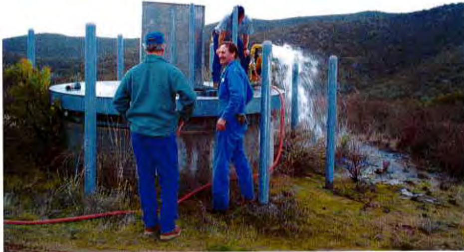
Maintenance Superintendent Larry Seifert, Plant Maintenance Technician David Renelle, and Distribution Technician Jim Marshall making repairs to an AVAR (Air Vacuum Air Release valve) near Santa Margarita – December 22, 2003.
