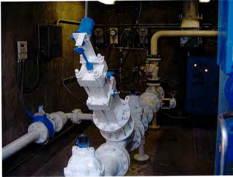
Sleeve valve controller at the Southern California Water Company Turnout.
