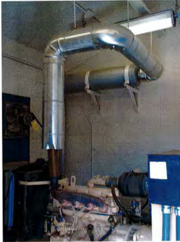
Standby generator at valve vault facility.
