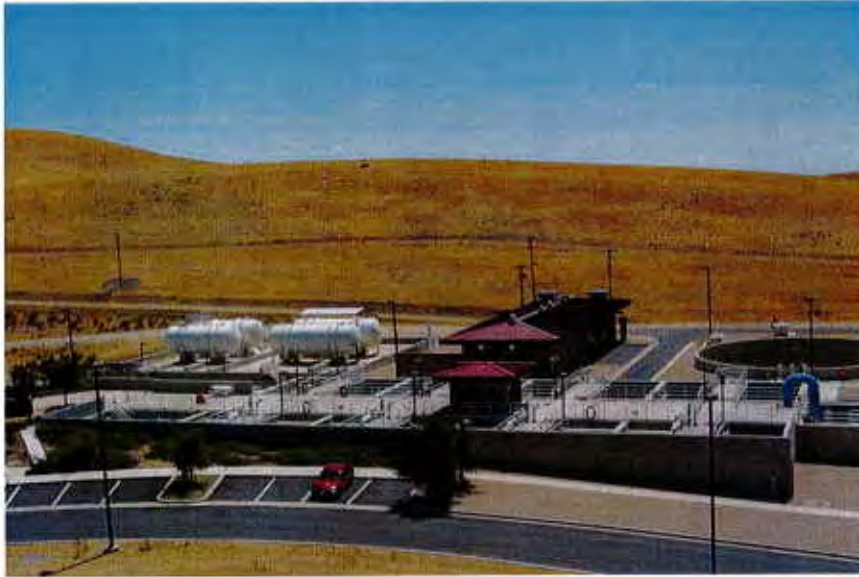
Polonio Pass Water Treatment Plant facilities showing dual media filters, chemical storage tanks, chlorine storage, and equalization tank.
