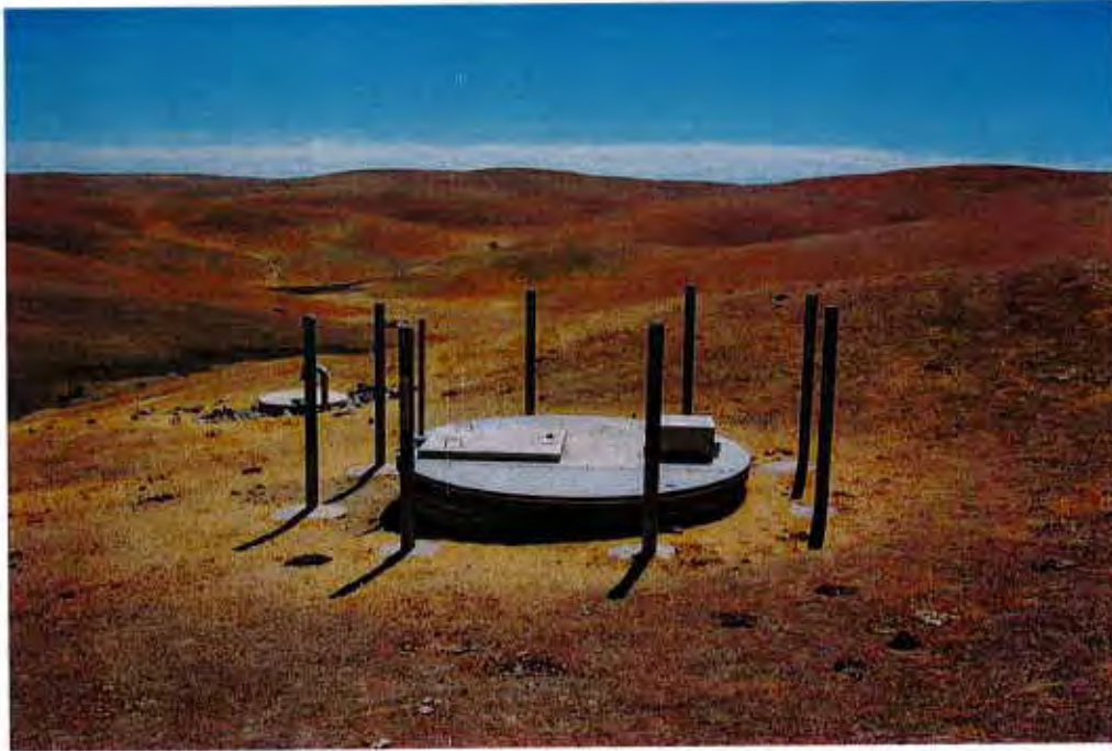
Reach 2 blow-off vault near Shandon, CA.
