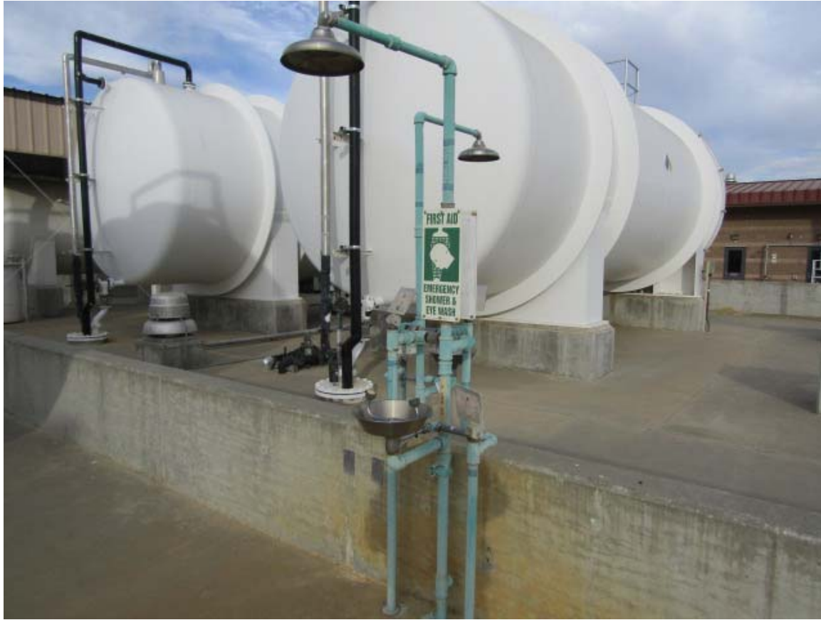
Eye Wash Station at Polonio Pass Water Treatment Plant
