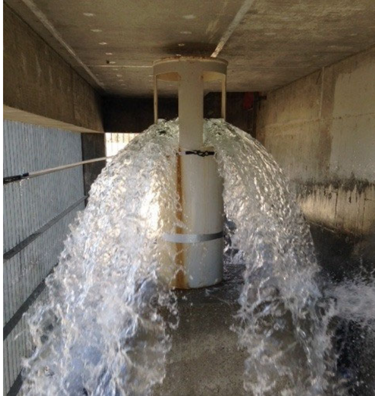
GTO Blow Off / Shutdown November 2022
