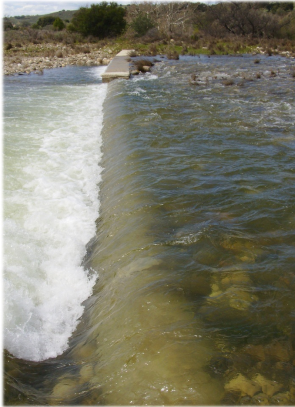
Santa Ynez River Pipeline Exposure
