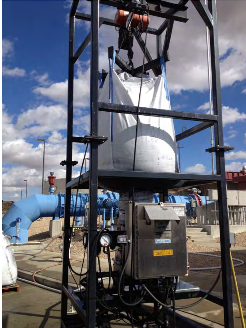
Powderf Activated Carbon (PAC) Vtgcw gpnUnit at Water Treatment Plant
