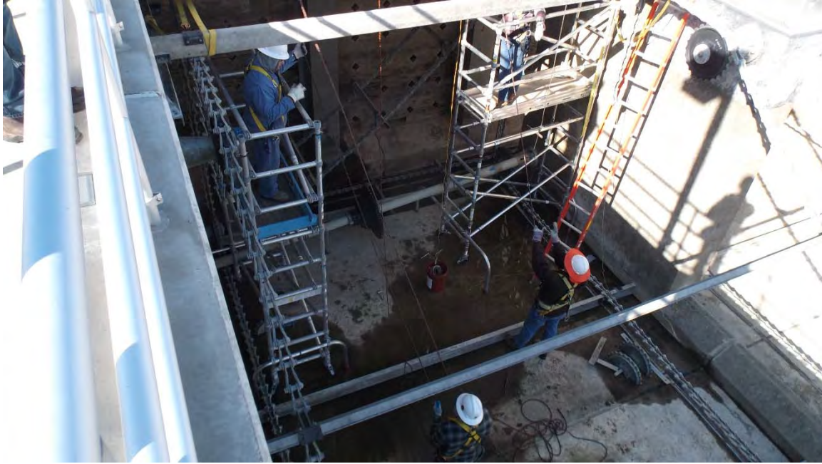
Maintenance and Distribution Crew Rebuilding One of the Sludge Collection Systems at Polonio Pass Water Treatment Plant
