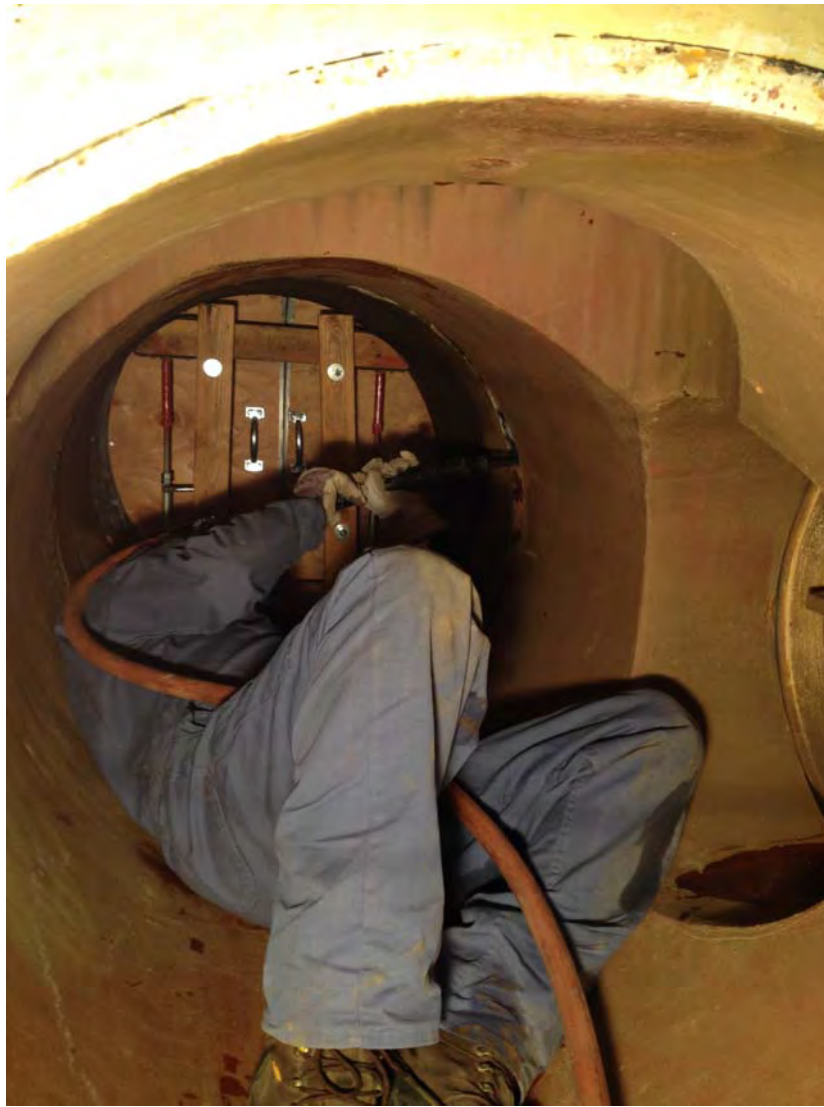
Repair of the filter effluent pipe internal protective coating during Winter Shutdown 2015
