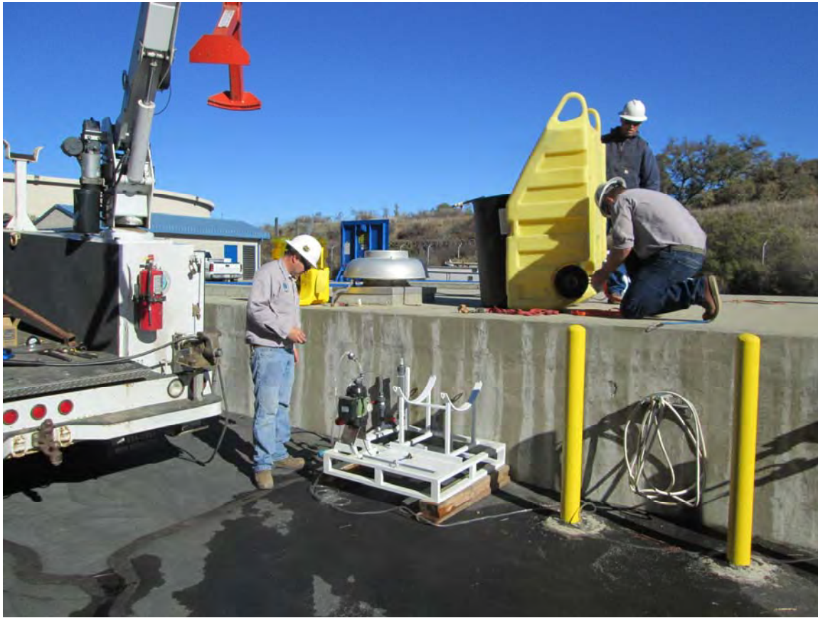
Tank 2 Chlorination during 2016 Winter Shutdown
