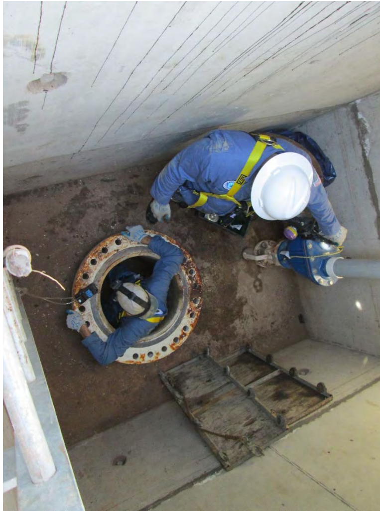
Internal inspection of the pipeline below the Thompson Avenue Cavity and the Willow Road Encasement
