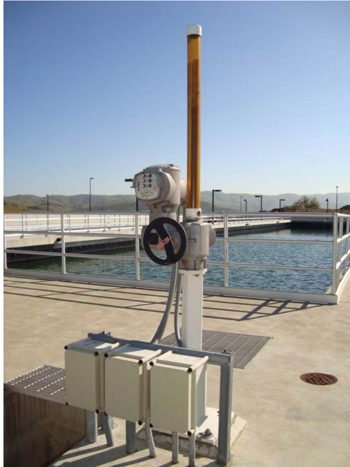
Telescoping valve for Sludge Removal System
