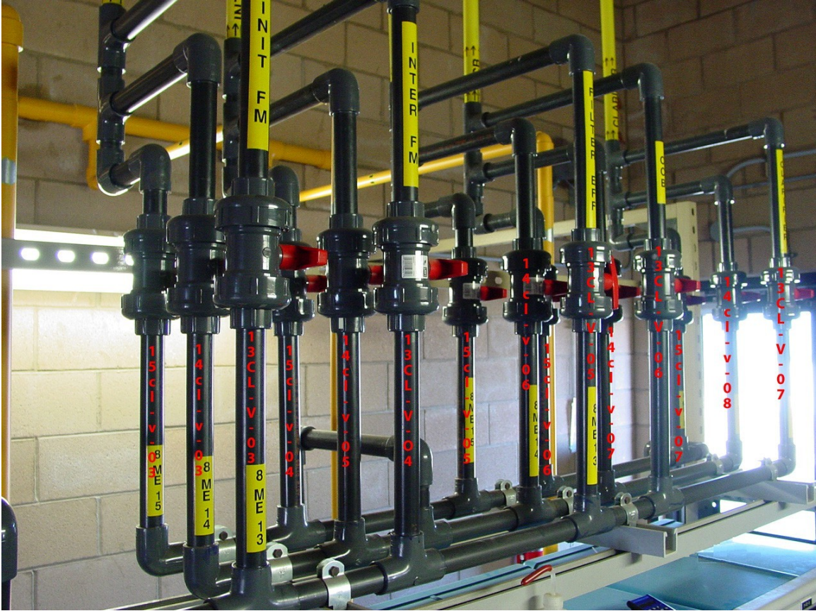
Chlorine Gas Manifold Piping in Chlorinator Room
