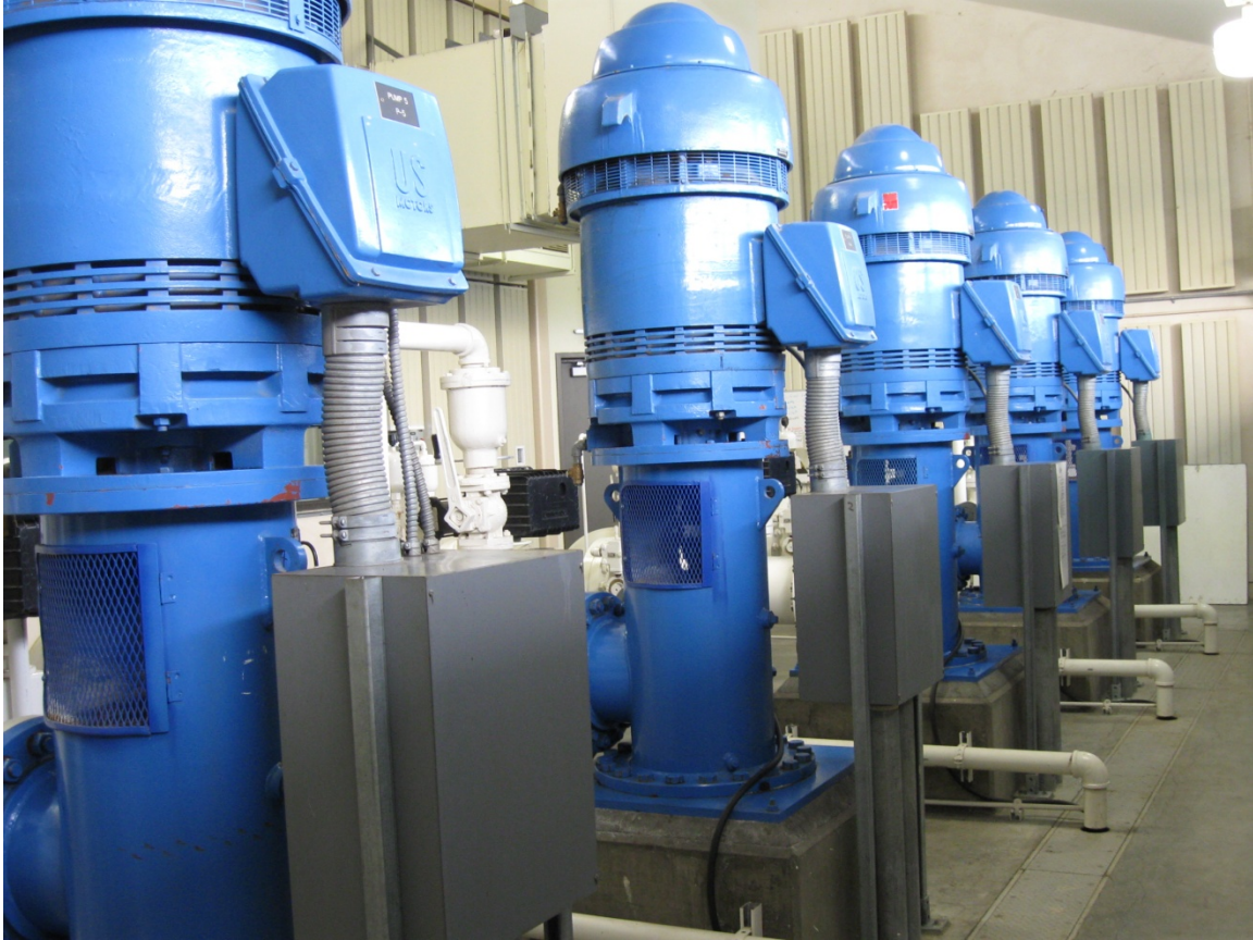
Santa Ynez Pumping Plant
