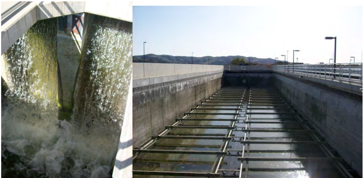
Floc/Sed basin refilling
