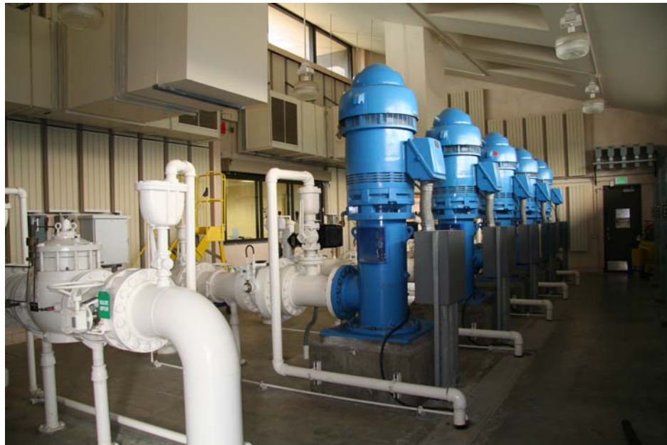
Santa Ynez Pumping Plant
