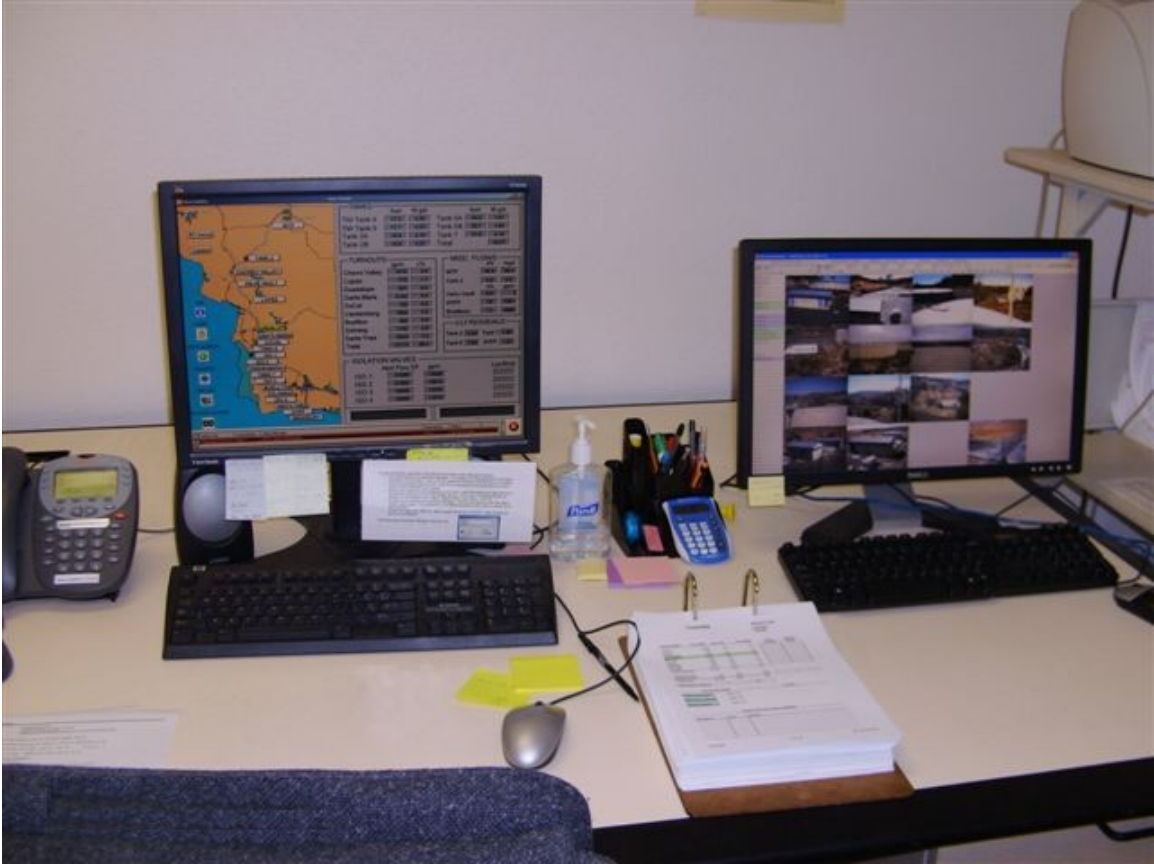
Distribution Control Room
