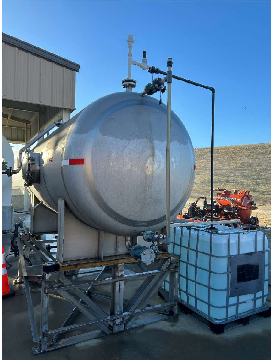
Ammonia Tank Transfer at Polonio Pass Water Treatment Plant
