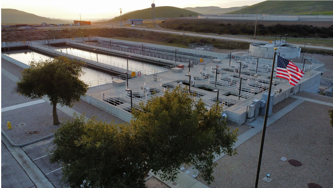
Polonio Pass Water Treatment Plant Flocculation/Sedimentation Basins.
