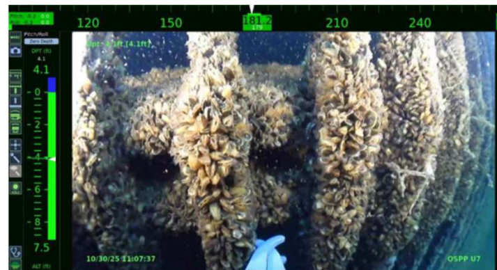
Oso Pumping Plant – Unit 7 Trash Rack
